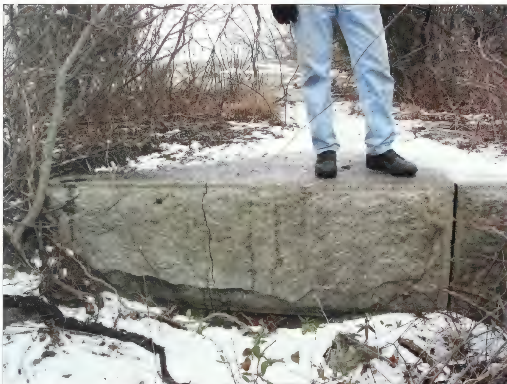
Figure 5.56. Portion of the northeast curtain wall belonging to the former granite fort. This large granite block is located north of gun platform #8. A longer section of the curtain wall and northeast bastion could be carefully exposed to help park visitors understand and appreciate the multiple layers of coastal defenses at Sandy Hook (Olmsted Center, January 2009).
